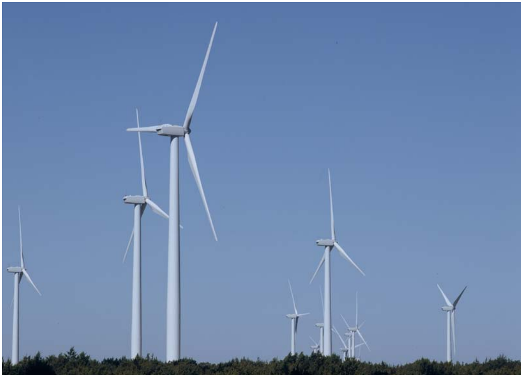
Wind Farm, Baldor motors are often used to control blade pitch and yaw
